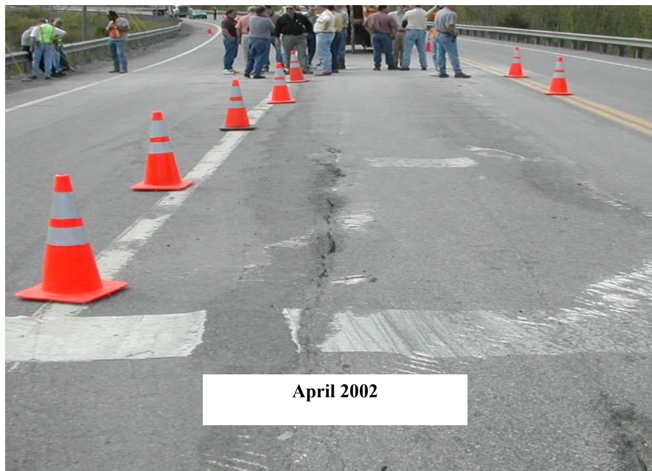
Figure 1.2 Condition of north bound approach on intersection
