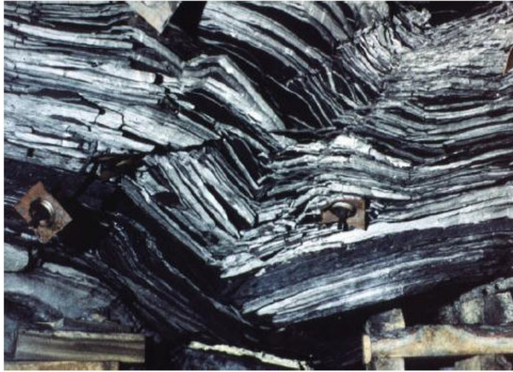
Figure 2.1 Cutter failure in thin beds of shale roof (Esterhuizen and Bajpayee, 2012)
