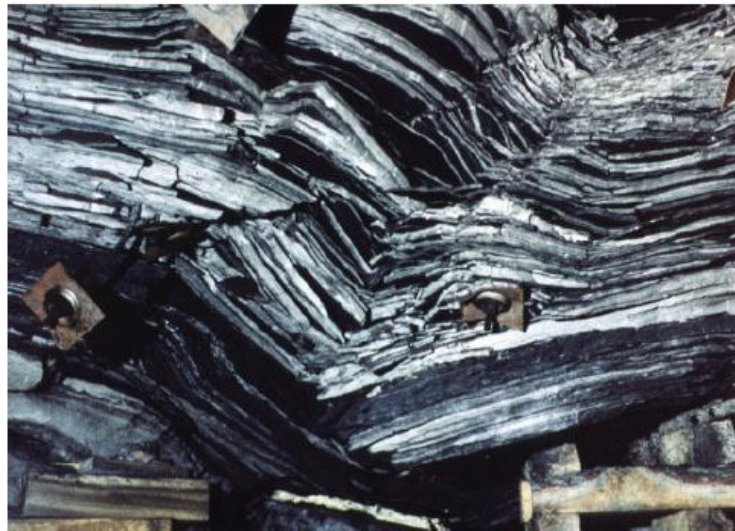
Figure 1.2 Cutter failure showing delamination in thin beds of shale roof (Esterhuizen and Bajpayee, 2012).
