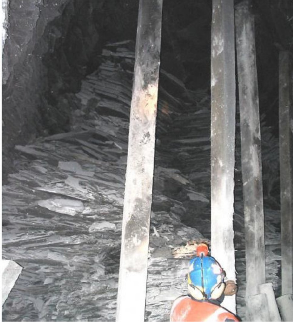
Figure 2.10 Result of progressive failure of laminated roof subject to high horizontal stress, the collapse has near vertical sides (Esterhuizen and Bajpayee, 2012).
