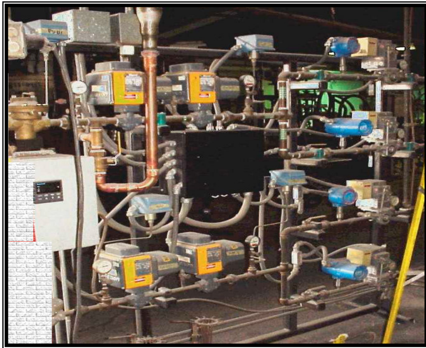
Figure 2.1 Picture of Pipe Trains
