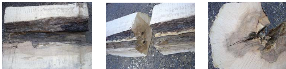
Figure 1-10 Decay or rot in wood
