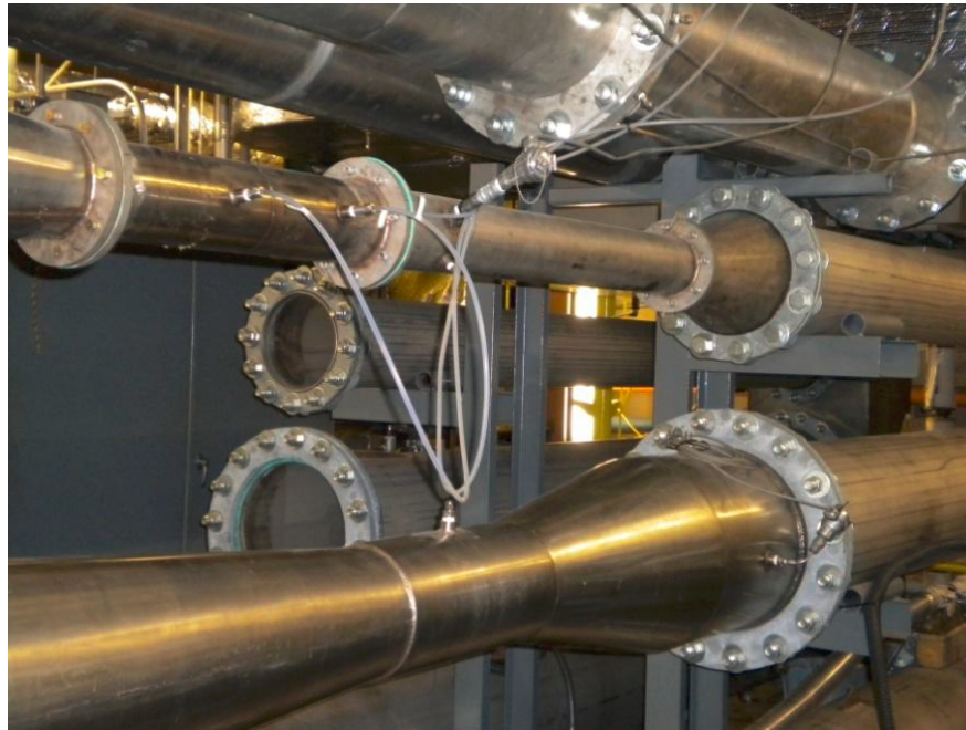
Figure 12: CVS tunnel in the EERL
