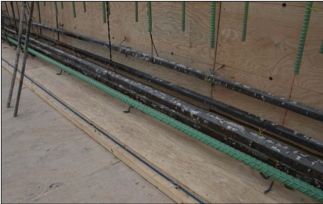
Figure 6.2 Missing Reinforcement Exposed in Beam 6
