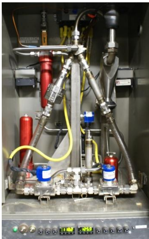
Figure 3.10 40 CFR § 1065 compliant PM sampling system at WVU CAFEE's EERL facility and on-board the TEMS
