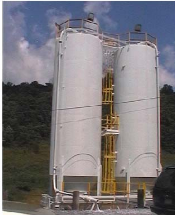
Figure 2.3 Photograph of Hydrated Lime Storage Vessels.
