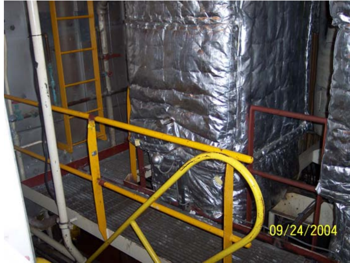
Figure 3-6 Exhaust Stack with SCR Catalyst
