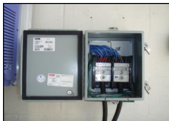
Figure 12: Terminal blocks splitting the energy from the Invertek drive unit to the immersion heater.
