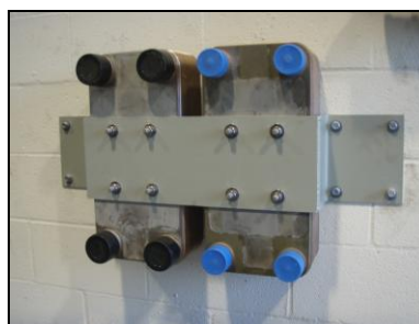
Figure 15: Wall-mounted flat plate heat exchangers.
