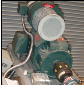
Figure 21: 40 horsepower A/C motor used for the SETC dynamometer.
