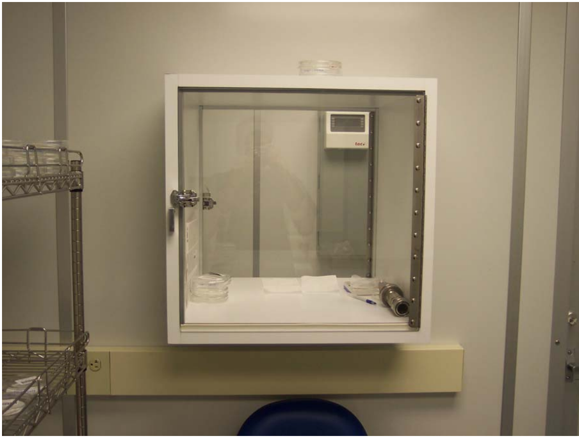
Figure 3-8: Pass through between cleanroom and gowning room
