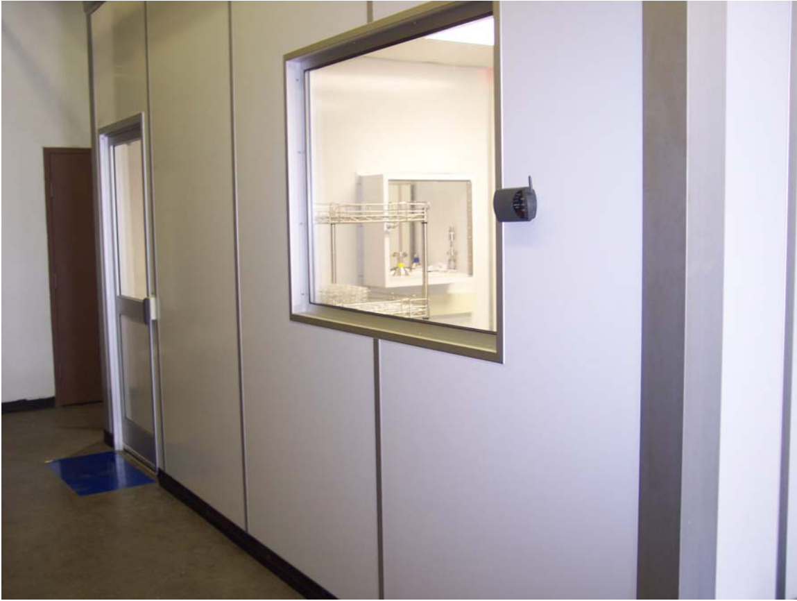
Figure 3-4: Outside view of cleanroom and gowning room
