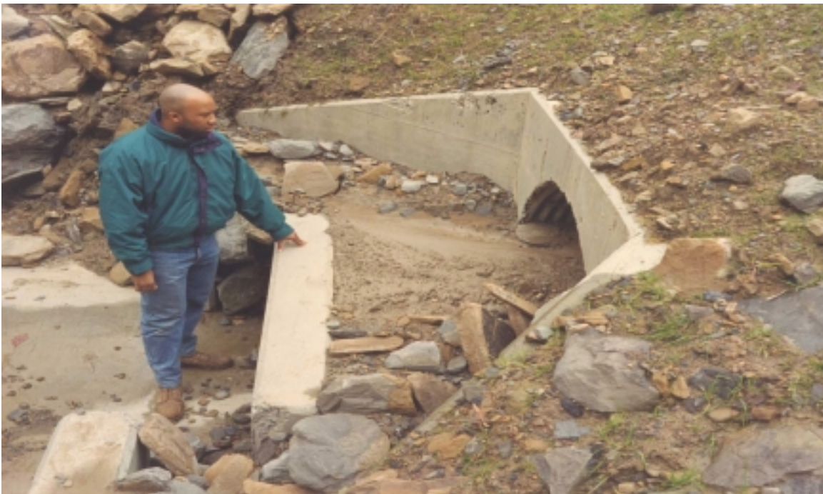
Figure 1.4.4 Failure of Baffle-type Energy Dissipator
