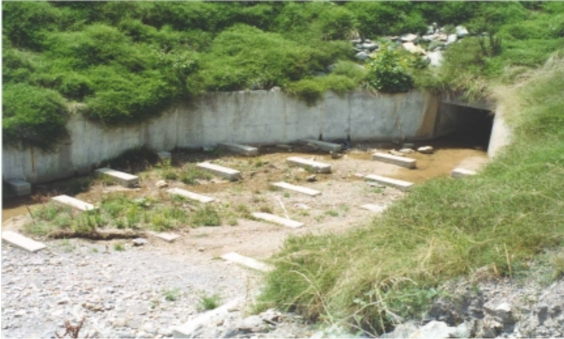
Figure 1.4.3 Failure of a Multi-Baffle Energy Dissipator
