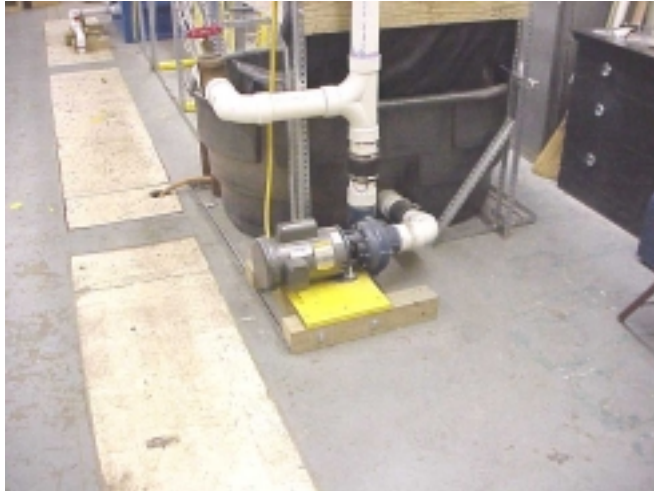
Figure 3.1 Centrifugal Pump Setup
