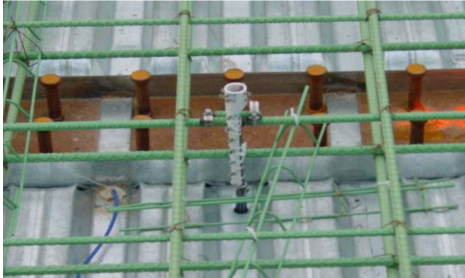
Figure 3.8: Thermistor Tree (photo courtesy of Dr. Shoukry, WVU)
