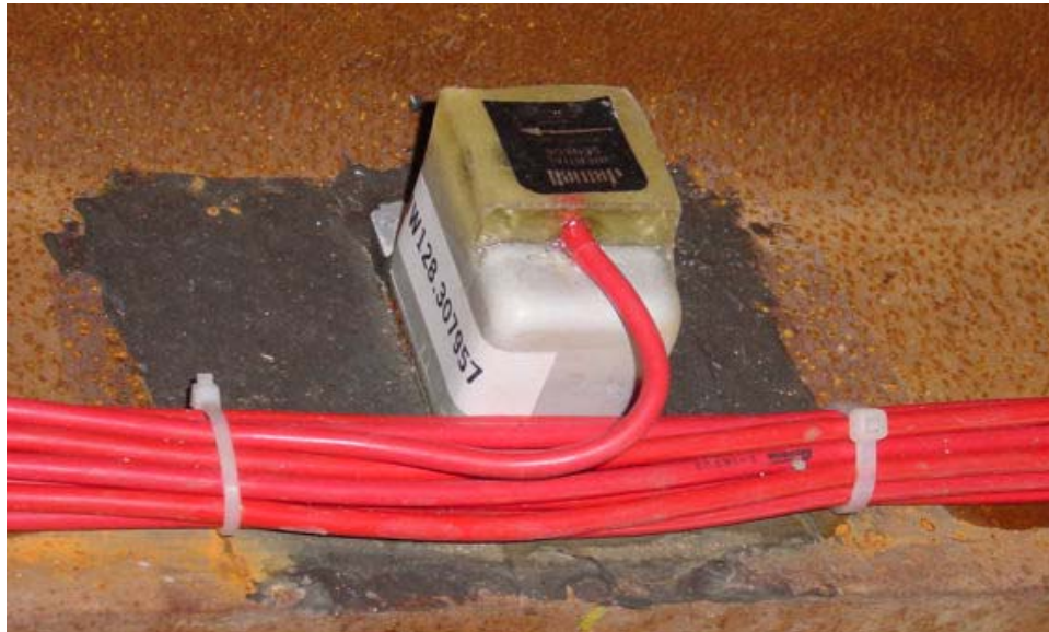
Figure 3.7: Inclinometer, Installed on Lower Flange of Girder B (photo courtesy of Dr. Shoukry, WVU)
