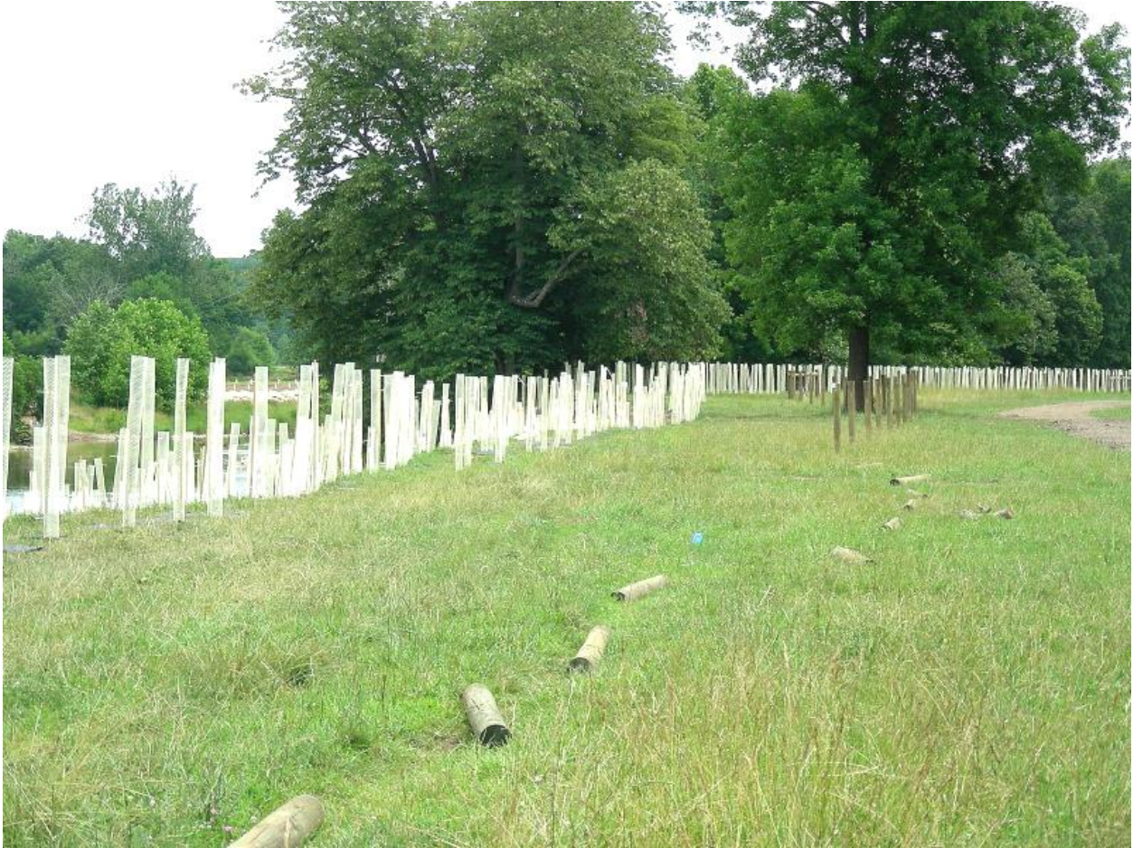
Figure 7. Construction of the barbed wire fence along the right side of the restoration reach. Thick posts are laying on the ground in the approximate locations that they will be placed, taken June 2010.
