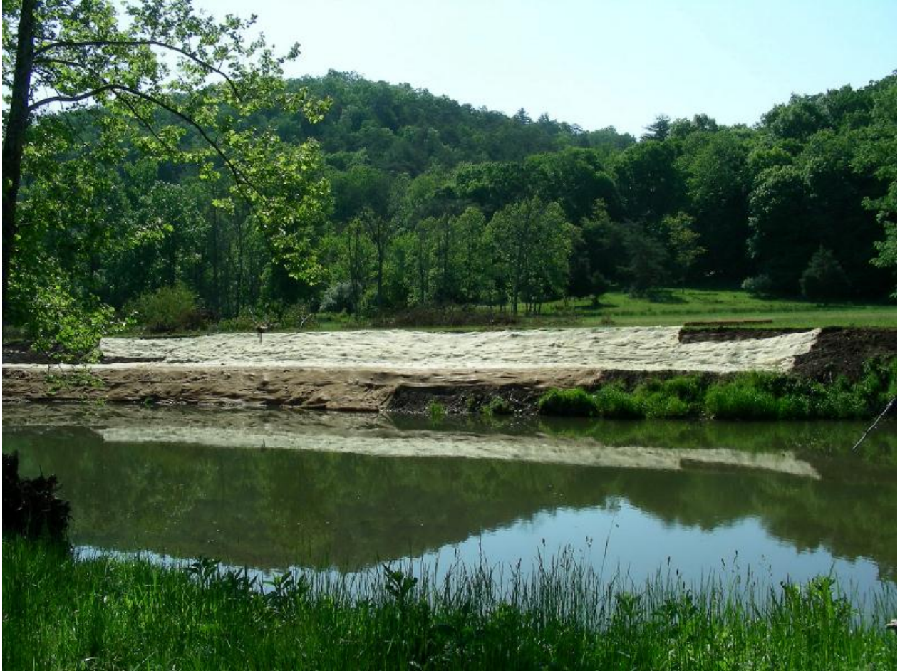
Figure 4. Geotextiles were laid down over the newly sculpted banks along the restoration reach to reduce sediment loss, taken May 2010.
