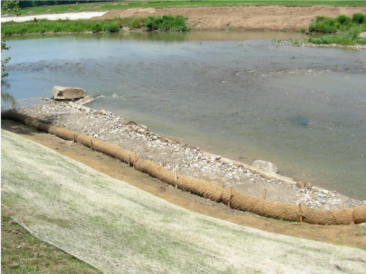
Figure 5. Log vanes were put into place along the restoration reach to deflect the main current from shore and decrease the erosion impact. The logs were anchored into the bank and held in place by large boulders. The inside angle was filled with streambed material. Coconut bio-logs were placed along the bottom of the contoured banks to catch sediment. The left side of the restoration reach is seen with newly constructed banks, taken June 2010.
