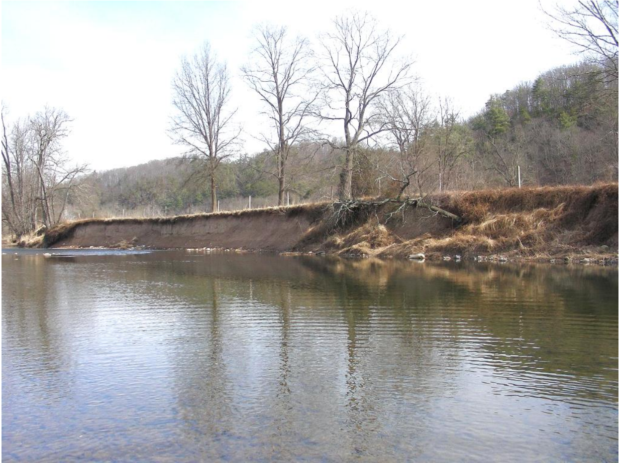
Figure 2. The right side of the restoration reach before restoration occurred, taken February 2009. The high, eroded banks with collapsing vegetation are clearly seen. The fence bordering the active pasture on the floodplain is at the edge of the streambank.
