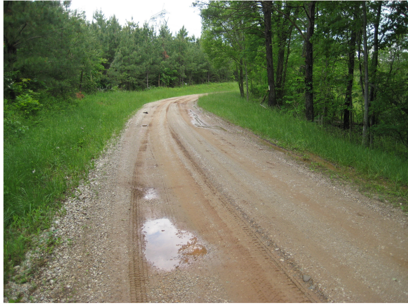
Figure 4.4 Rutting and Potholes on Oak Grove Road Prior to Road Maintenance
