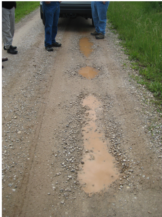
Figure 4.5 Potholes on Oak Grove Road Prior to Road Maintenance
