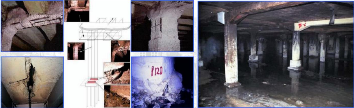
Figure 82: Safety problem in structure portion (source: Cheong Gye Cheon Restoration Project, 2006)
