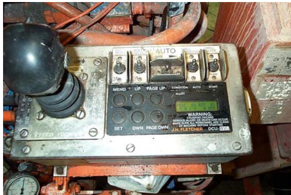
Figure 4.8 Joystick on Control Panel
