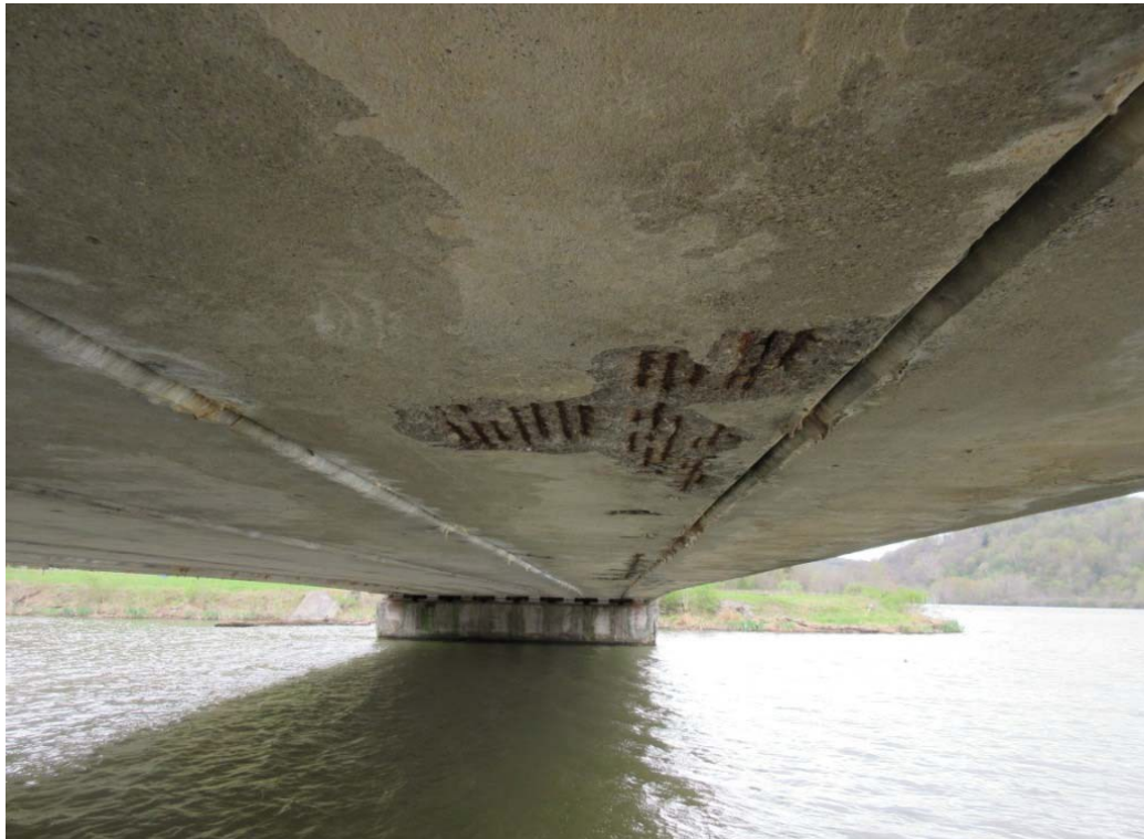
Figure 5-3: Main Span Beam - Exposed Strands (Kollias 2015)
