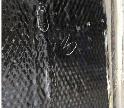
Figure 5-18: Debond 8-3 with two small pockets on Beam 8 of Whiteday Bridge
