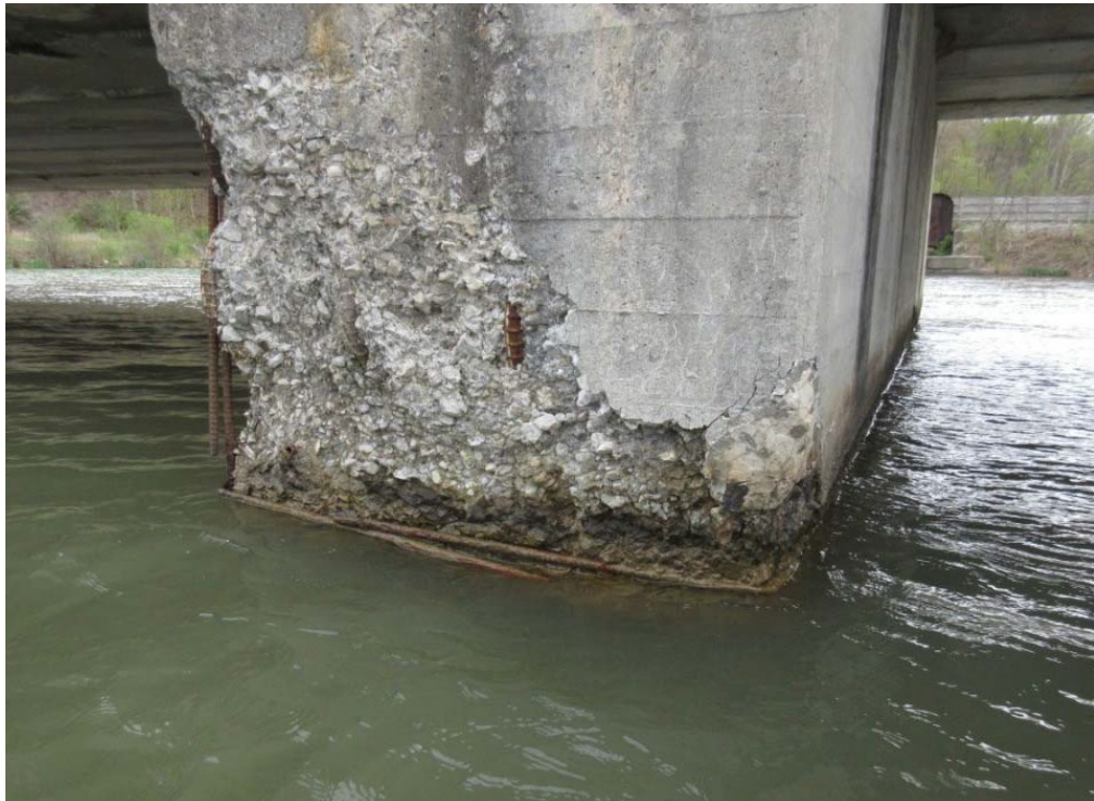
Figure 5-7: Concrete spalling at the surface of contact with water in Pier 1 (Kollias 2015)
