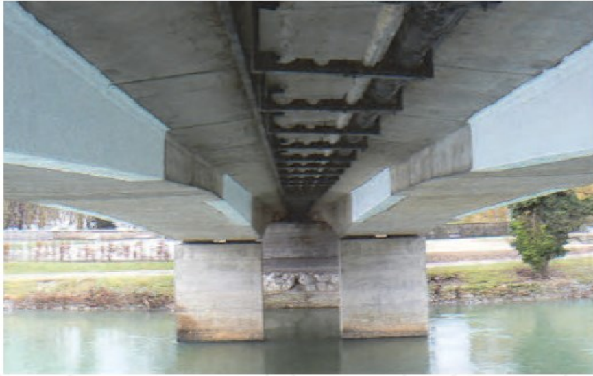
Figure 3-10: FRP Strengthened Box-Girders of the Bridge (Taillade et al. 2012)
