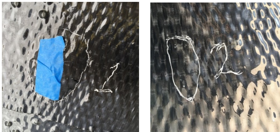
Figure 5-13: Defective Spots 1-1 (left) and 1-2 (right) on Beam 1 of the Whiteday Bridge
