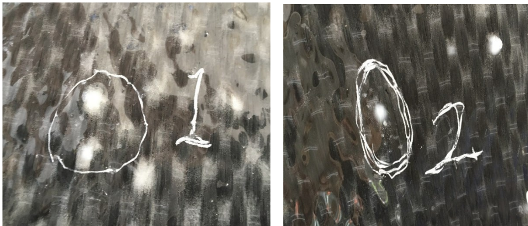
Figure 5-15: Defective Spots 4-1 (left) and 4-2 (right) on Beam 4 of the Whiteday Bridge
