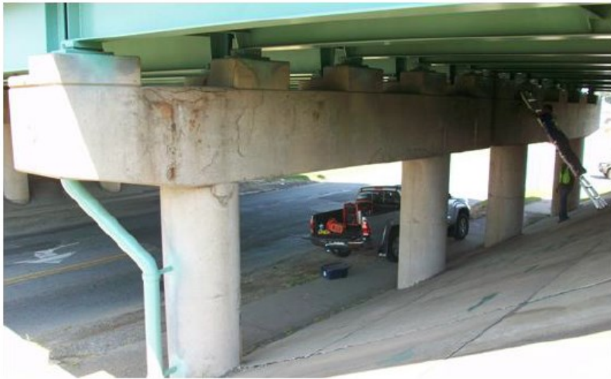
Figure 3-3: Close-up view of the damaged piers and pier cap on the south side of the bridge (Halabe et al. 2012)
