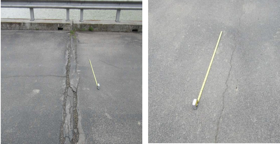
Figure 5-4: Heaving on the wearing surface at Pier 2 deck joint (left) and Longitudinal cracks (right) (Kollias 2015)
