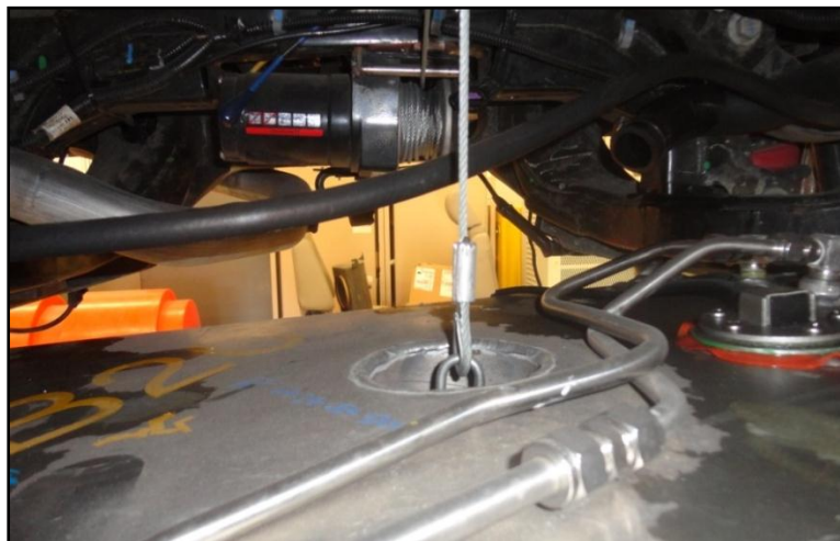
Figure 58. Fuel Tank Winch Cable Attachment
