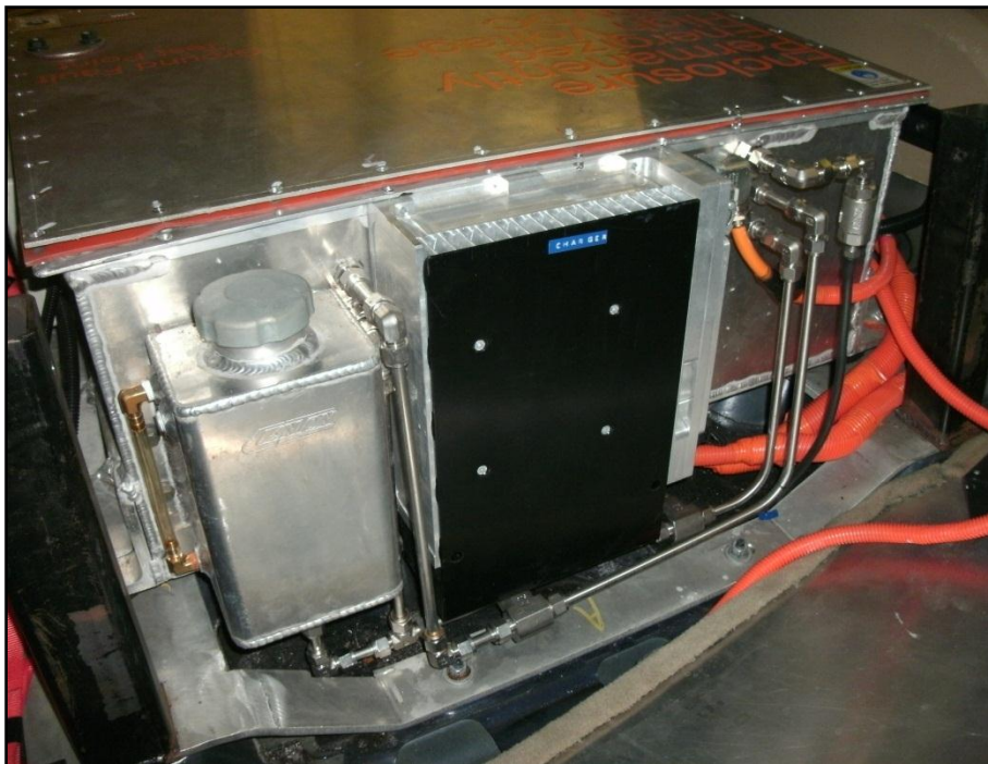
Figure 47. Front of High-Voltage Battery Enclosure
