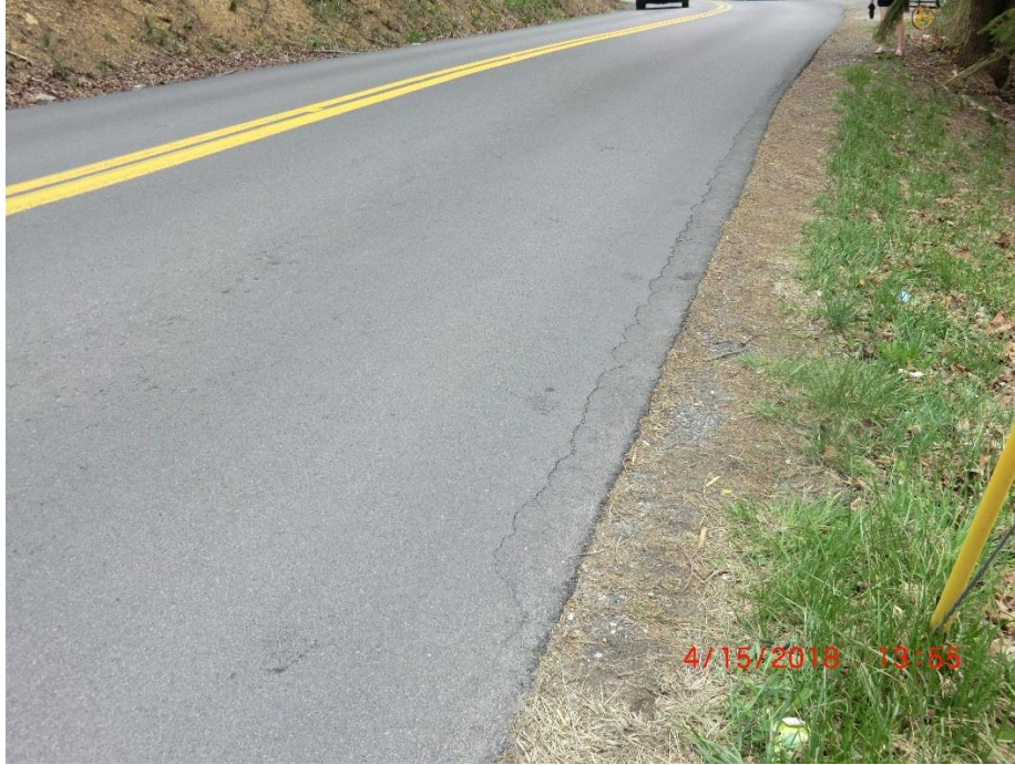
Figure 14: Edge Cracking in the Wearing I Section
