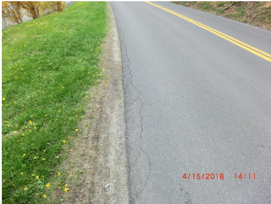
Figure 15: Edge Cracking in the Wearing I with FORTA-FI Section
