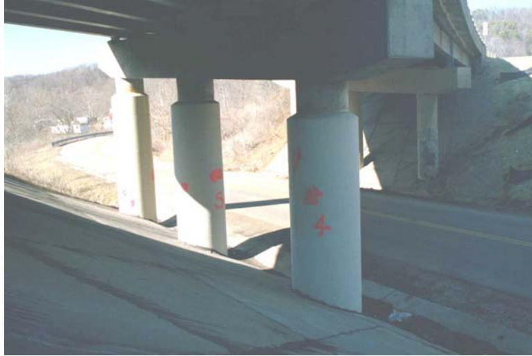
Figure 5.4.3. Delaminations found by tap testing of three pre-cured shell wrapped columns.
