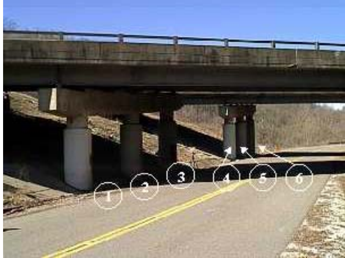
Figure 5.2.2. Photographic view of the Pond Creek bridge. The columns marked 1, 2 and 3 are wrapped by hand lay-up method and those marked 4,5 and 6 are wrapped with pre-cured shells.
