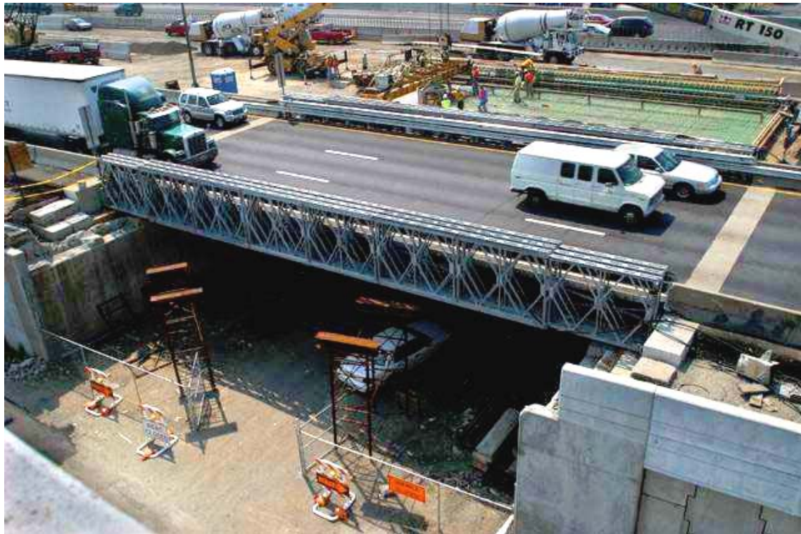
Figure 4-47 Acrow Panel Bridge [21]
