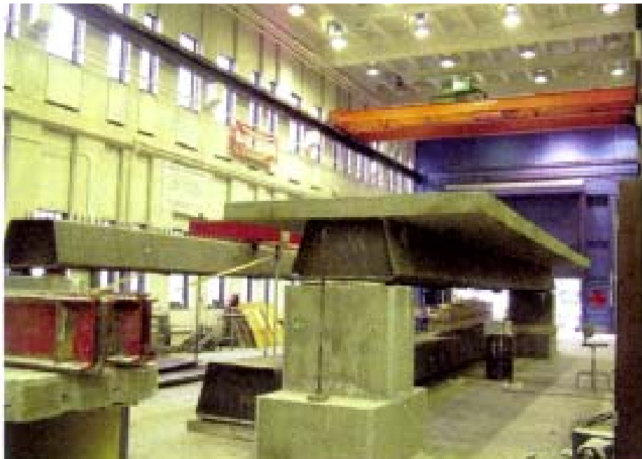
Figure 4-41 Section of Folded Plate Girder Bridge Ready to be Stacked and Shipped [8]
