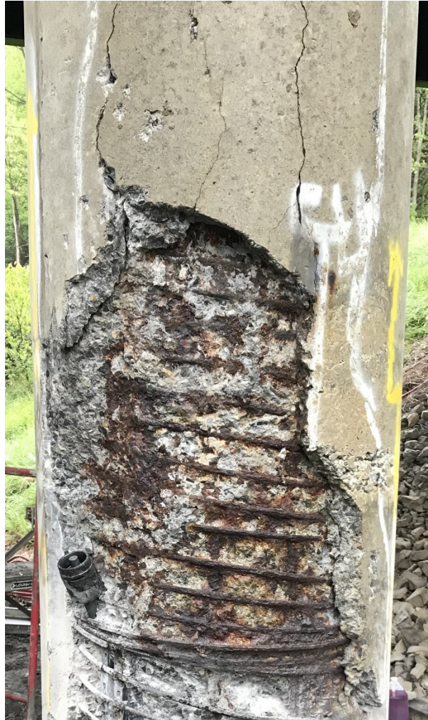
Figure 3.3: Concrete spalling on pier 3.
