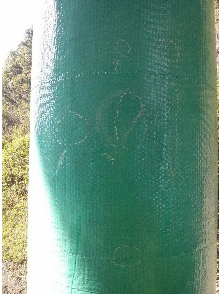
Figure 4.18: Debonds found in the west column of pier 1.
