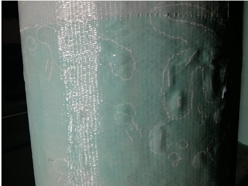
Figure 4.22: An example of the amount of debonds found while testing columns pier 2.
