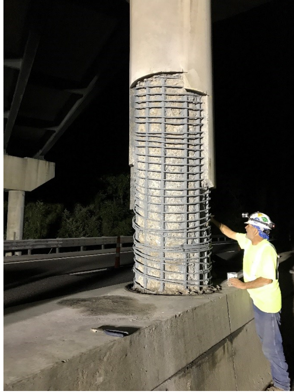
Figure 4.21: West column of pier 2 while corrosion inhibitors were being placed on the rebar.
