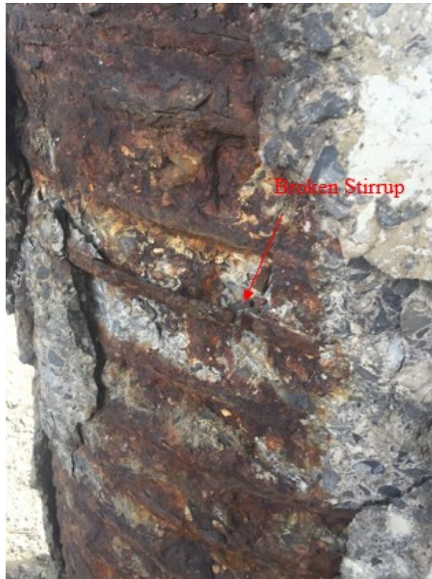
Figure 4.4: Corrosion of the stirrups on one of the columns.
