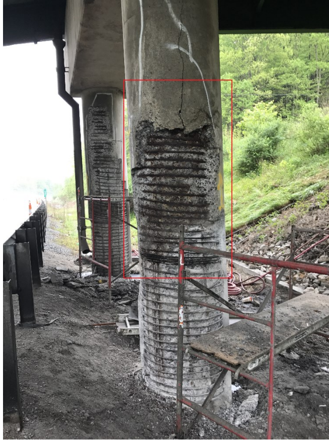
Figure 3.2: Extent of original concrete spalling.
