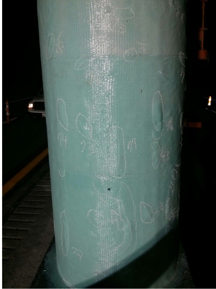
Figure 4.23: The lower half of the west column on pier 2 and debonds that were found.
