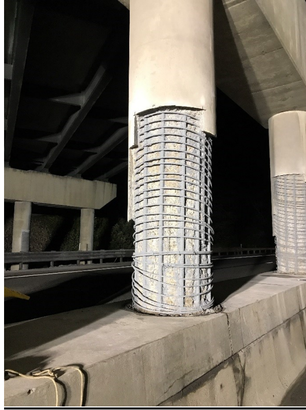
Figure 4.20: Center column of pier 2 in the process of being prepped for concrete repairs.
