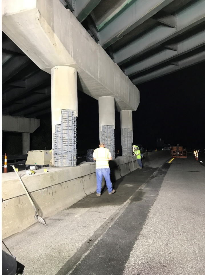
Figure 4.19: Image showing all three columns of pier 2 and the necessary concrete repairs being made.
