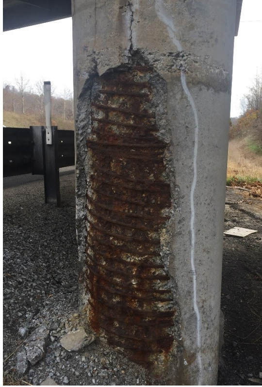
Figure 4.3: Concrete spalling prior to rehabilitation.
