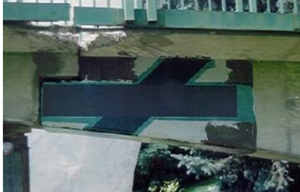
Figure 2.39: CFRP sheets applied in the horizontal and diagonal direction (Hutchinson et al. 2003).
