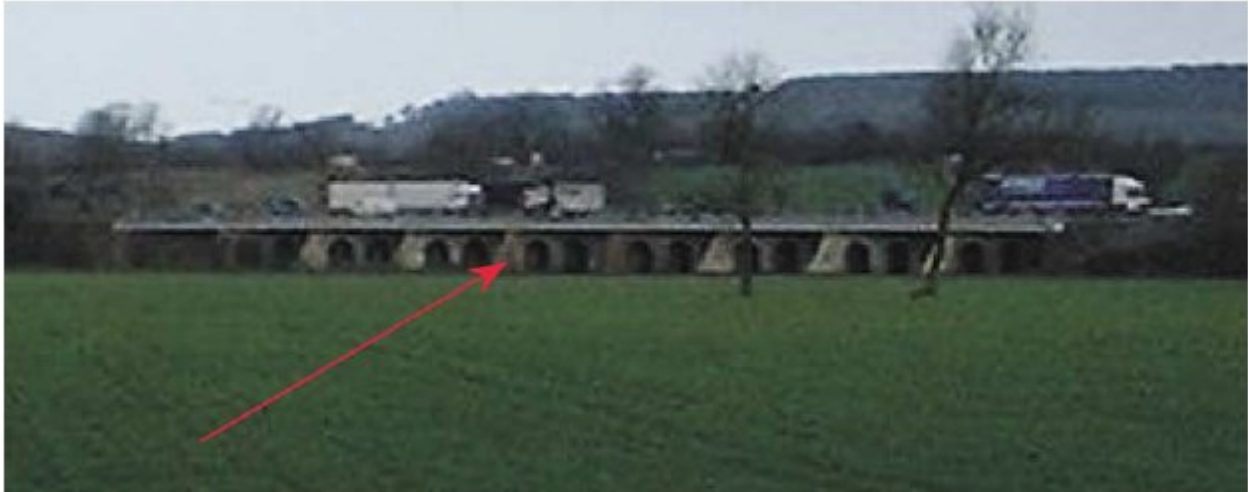
Figure 2.7: Photo of the bridge being studied with an arrow pointing to span 5 (Clark et al. 2003)
