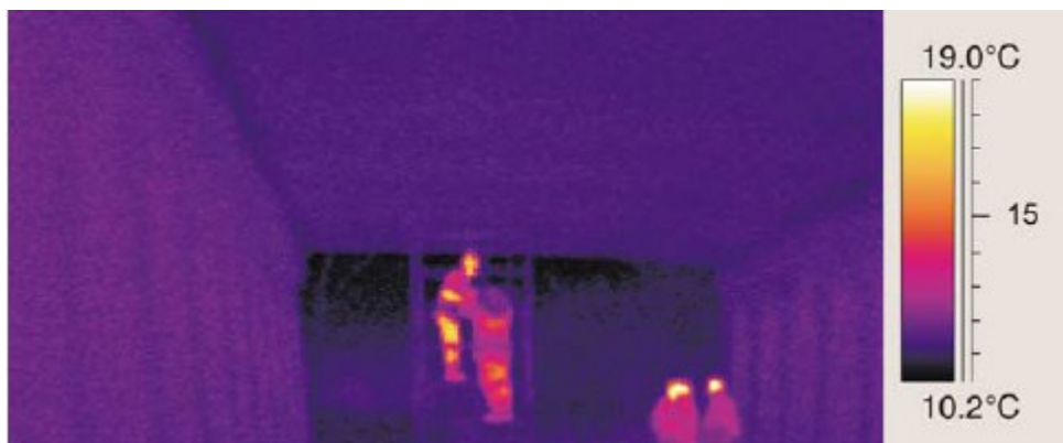
Figure 2.8: Infrared image looking down span 5 with all temperatures considered (Clark et al. 2003).
