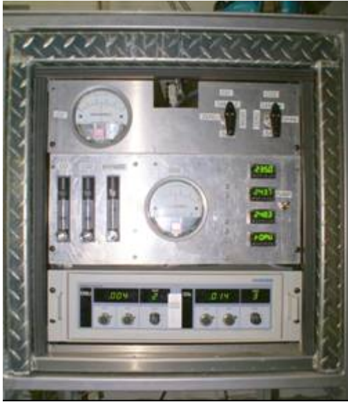
Figure 19 - NDIR Analyzer for CO and CO 2
