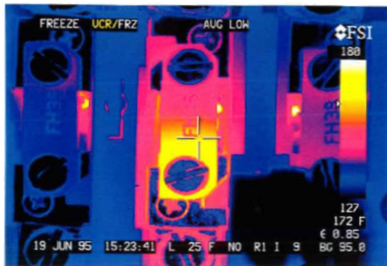
Figure 2.3: Infrared image for excessive heating of a connecting clip [13].
