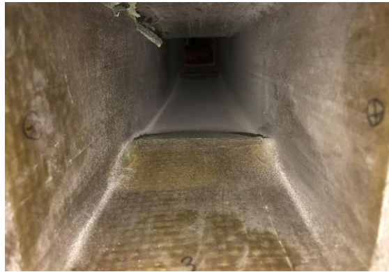
Figure 7-61. Transverse shear failure in bottom flange on HWB beam over the support
