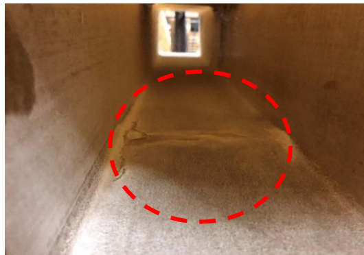
Figure 7-57. Bottom flange fracture on CB beams over the support
