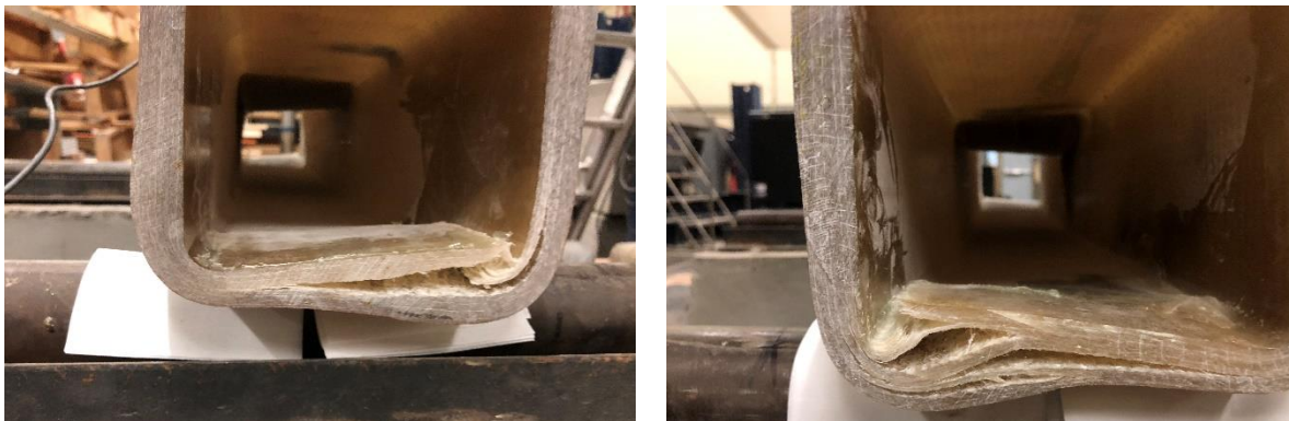
(a) (b) Figure 7-49. Failure at the support regions, (a) delamination, (b) delamination and warping
