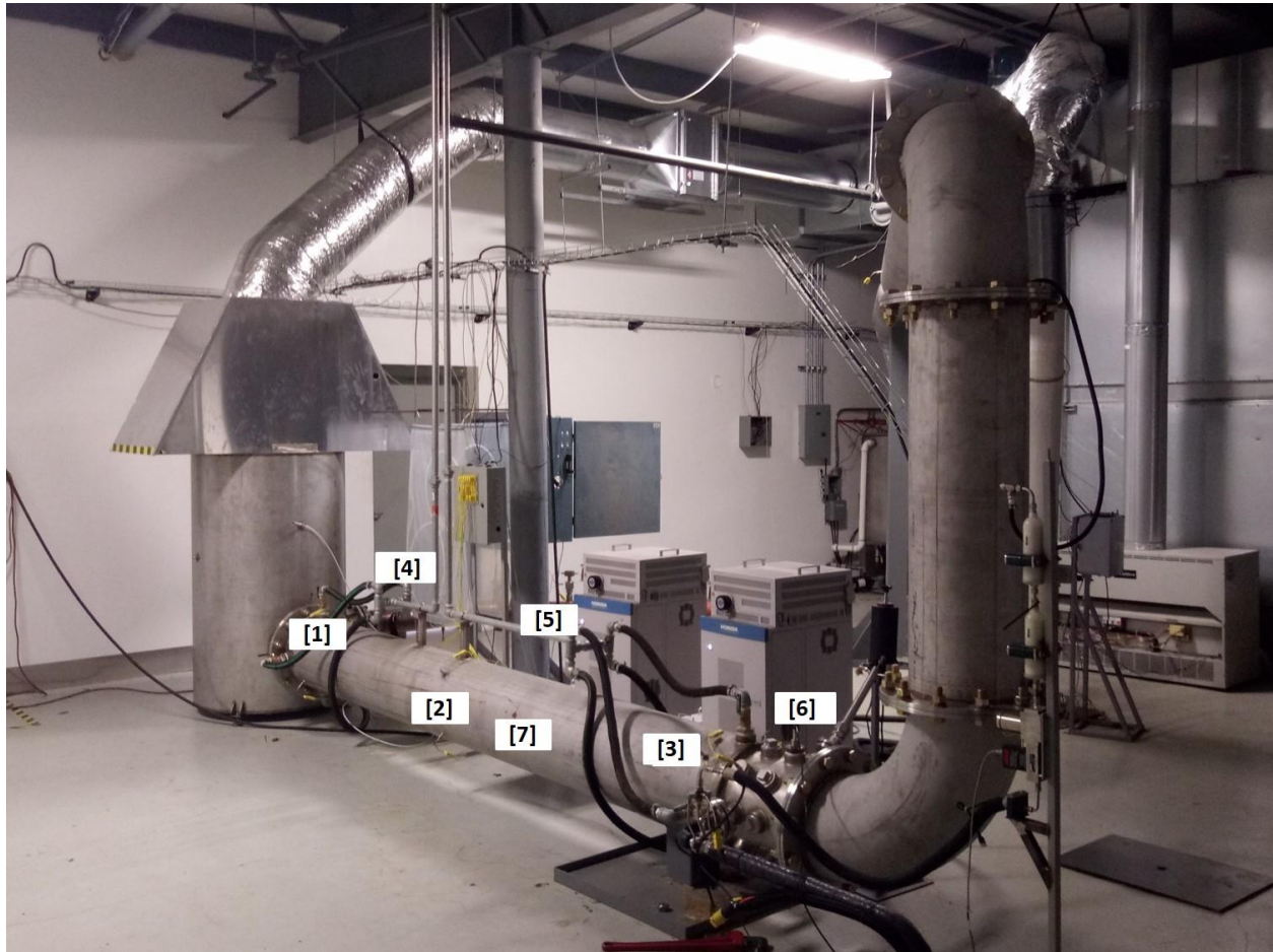
Figure 19- Tunnel Heating Set-up: Thermocouples locations [1,2,3], Dilution air and exhaust mixing chamber entrance [1], Hot water inlet [4], Water Outlet [5], Sampling Plane [6], Tunnel Heating Jacket [7].
