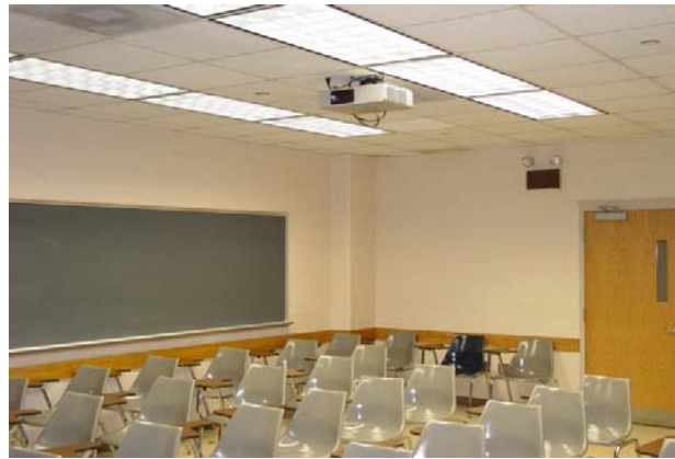
Figure 10.1 Lighting in MRB # 107
