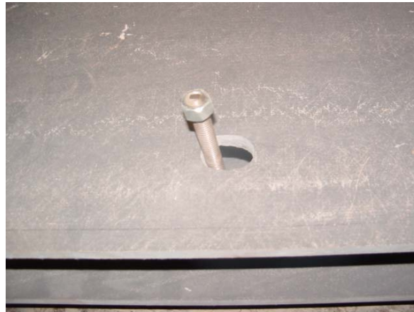
Figure 5.5: Diameters of holes were larger than that of threaded rods.
