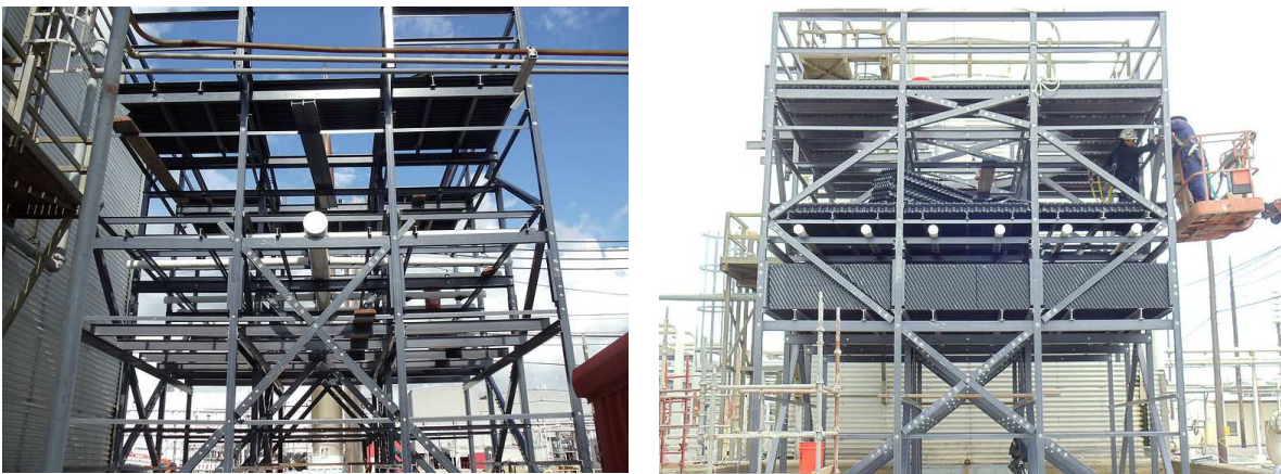
Figure 2-5: FRP Cooling Tower Structure (from Cooling Towers of Texas)
