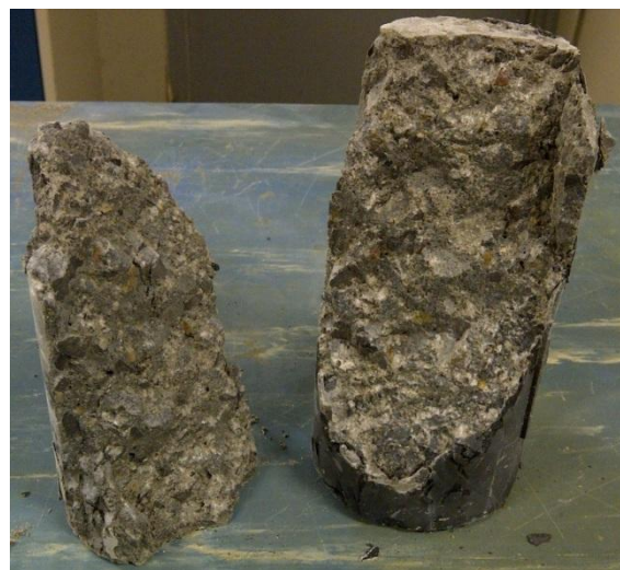
Figure 6.29 Failure through substrate
