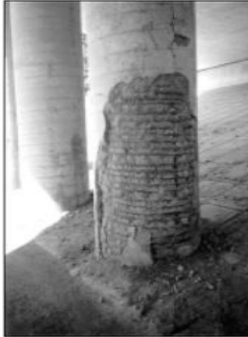
Figure 1.3 Deterioration of bridge pier
