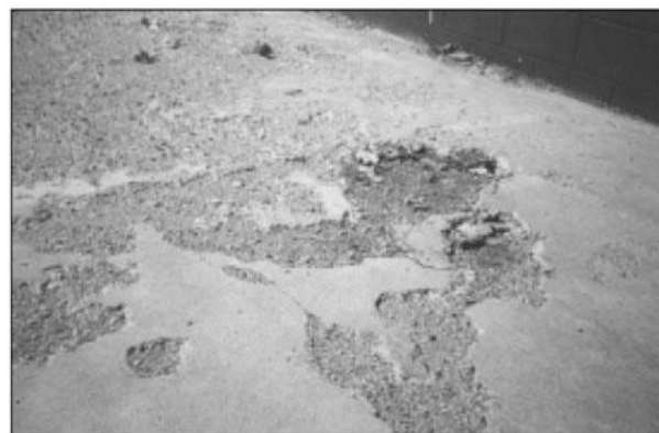
Figure 1.2 Deterioration of concrete deck
