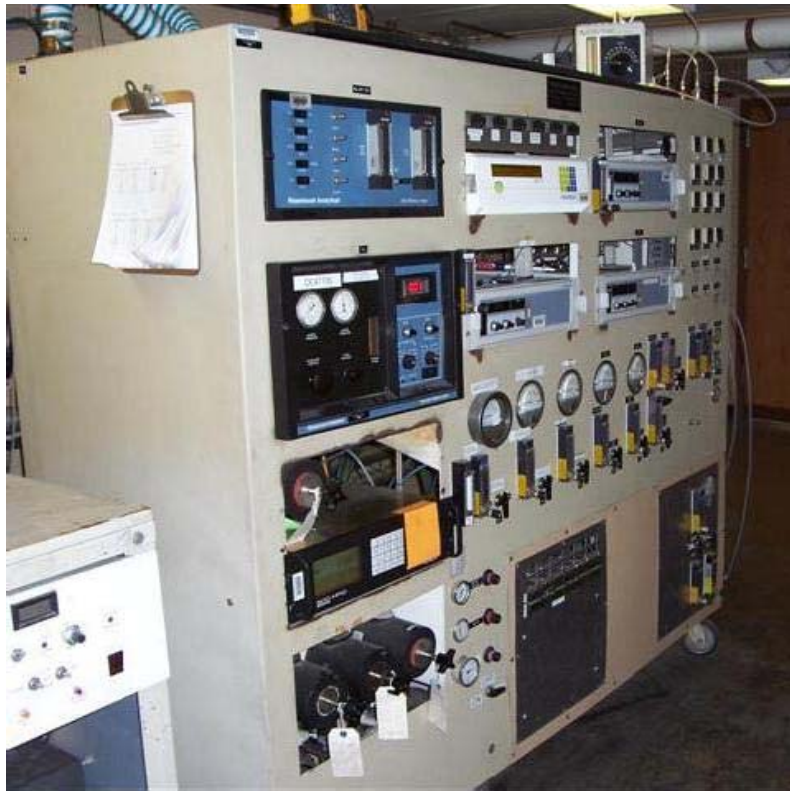
Figure 3- 1 Exhaust Analyzer Bench
