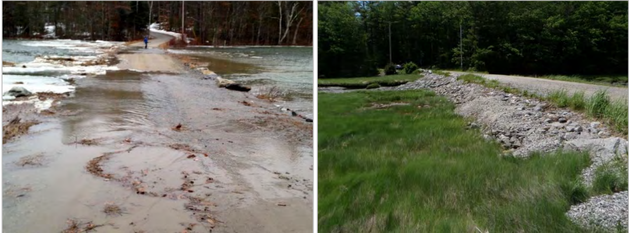
Figure 3. Photo-documentation of road overtopping and associated erosion of road material.
