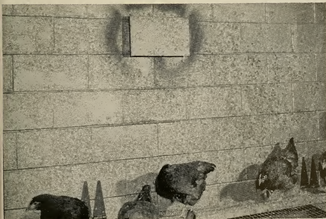
FIGURE 2. Flat plate baffle over the inlet of the wall helped to keep the wall dry, but did not direct the air over the birds and litter.
