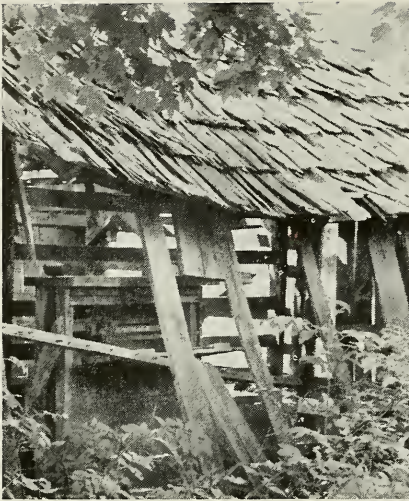
Fig. 10—Abandoned Country Weighing Facilities of Local Livestock Dealers
