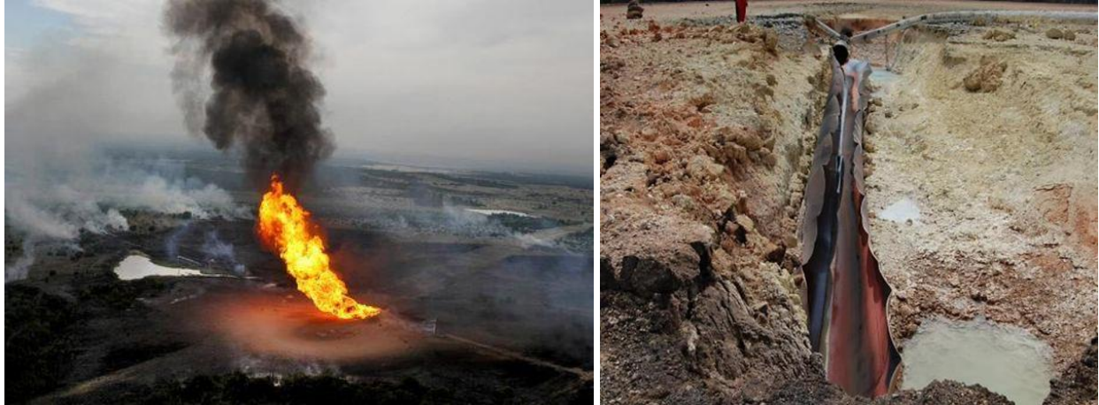
(a) Natural gas burning from 36" diameter pipeline (b) Ruptured section of the pipeline
