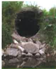
Combined sewer overflow
