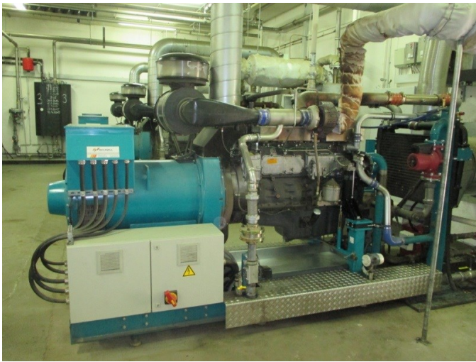
Fig. 2. Demonstration of a co-generation unit in the BS 1 biogas station
