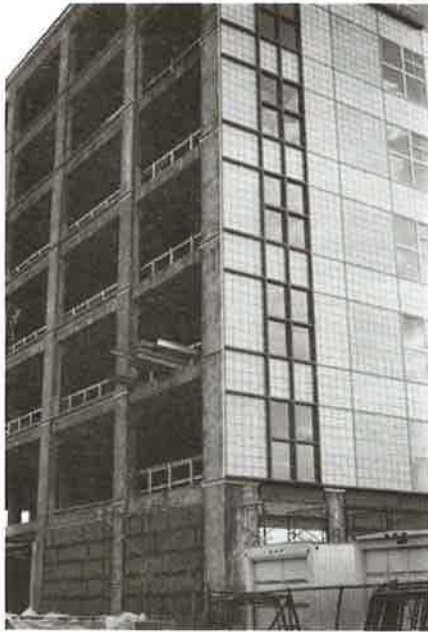
The Glickman Family Library as it looked when original renovations were underway. Now USM will finish the top three floors.
