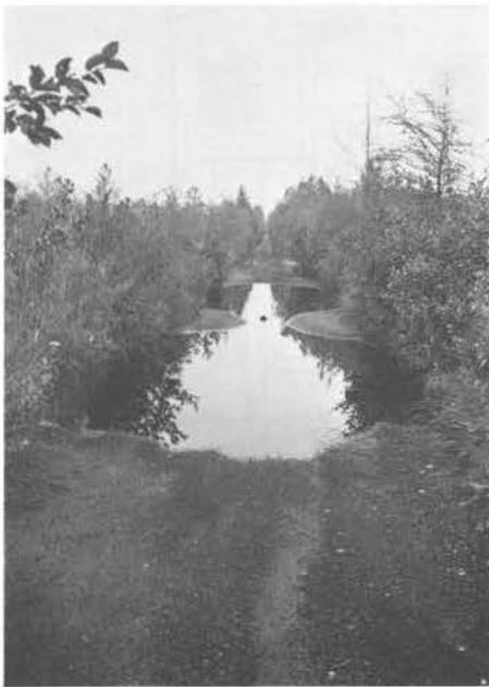
ABANDONED GRADE POORLY DRAINED
