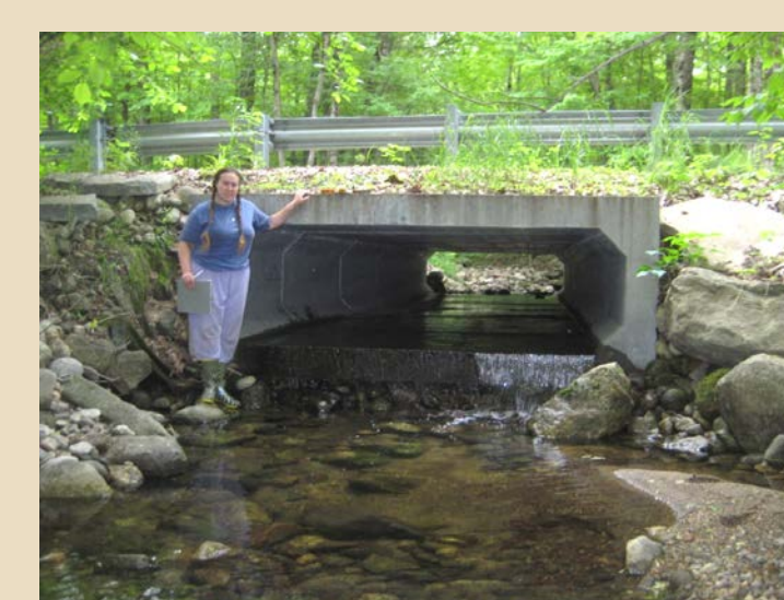
Photo 3. A perched culvert.
