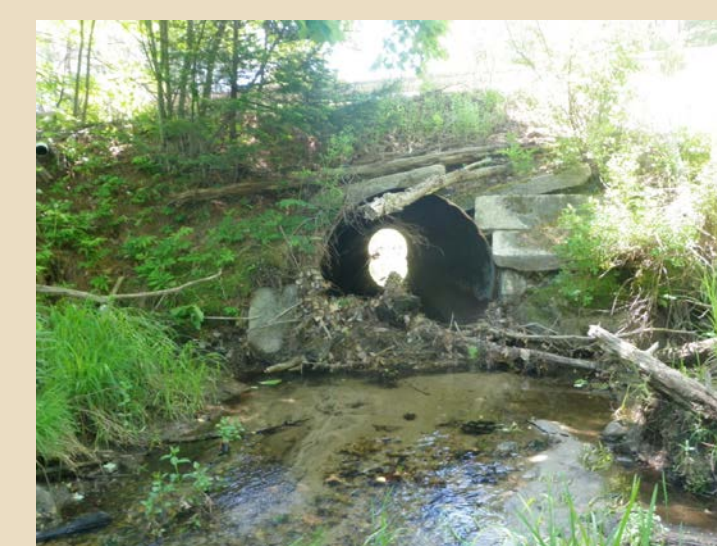
Photo 2. A partially blocked culvert.
