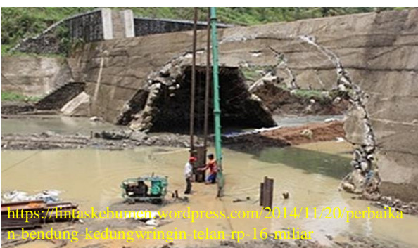
Gambar 5. Dam Kedungwringin jebol
