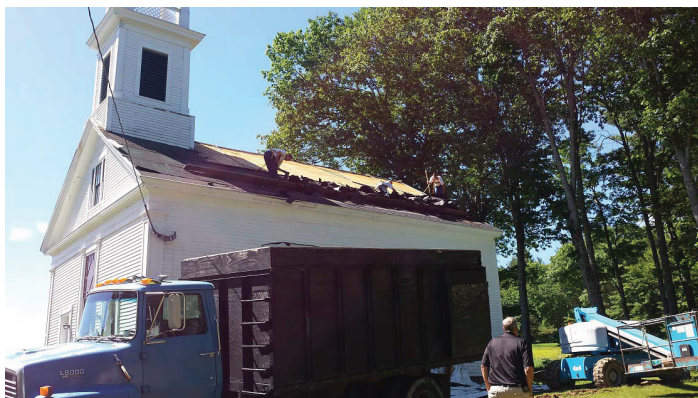
CO/CTI Chris Dutil's work crew strips shingles off the East Sangerville Union Church.
