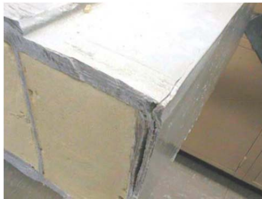
Figure 2: Voids resulting in surface cracks (Ryan et al [3])
