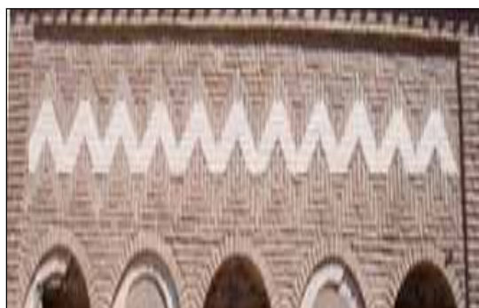
Figure 34: Zigzag lines in brick works
