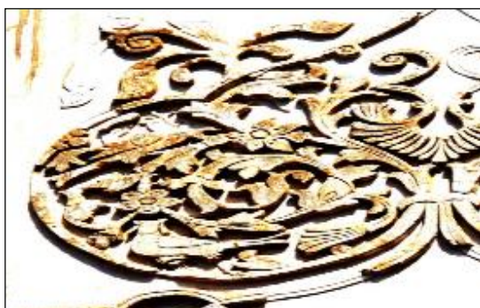
Figure 33: Bent lines in stuccos
