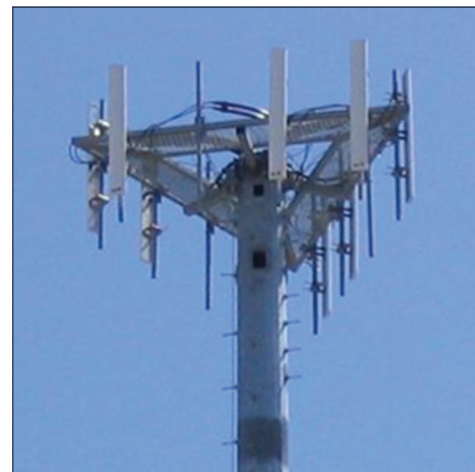
Figure 2. Top of a cellular radio tower. Nine sector antennae of three operators, three per one operator. http://en.wikipedia.org/wiki/Cellular_network
