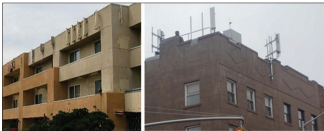
Figure 4. Photos show two examples of using cellular antennae that do not consider the safety guidelines (IEEE, 2006; FCC, 1997; ICNIRP, 1998) and distort the landscape.
