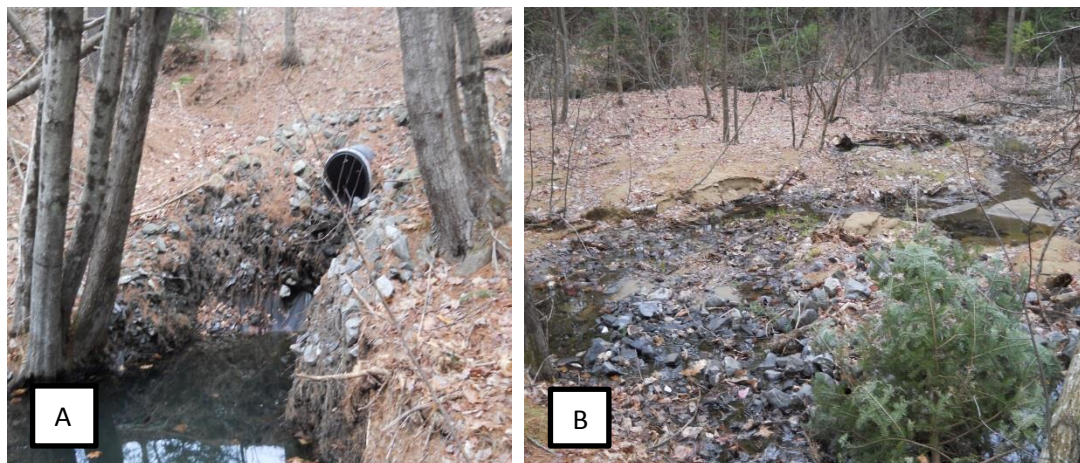
Figure 3: 3A: Scour at outlet of stormwater drainage; 3B: additional erosion and deposition of sediment downstream of the outlet shown in 3A. Note the rock washed out of the plunge pool at the outlet scattered down slope toward and in the eroded channel, suggesting that the outlet may be experiencing higher flows than anticipated in the design. Main channel of Topsham Fair Mall Stream is visible in the background.
