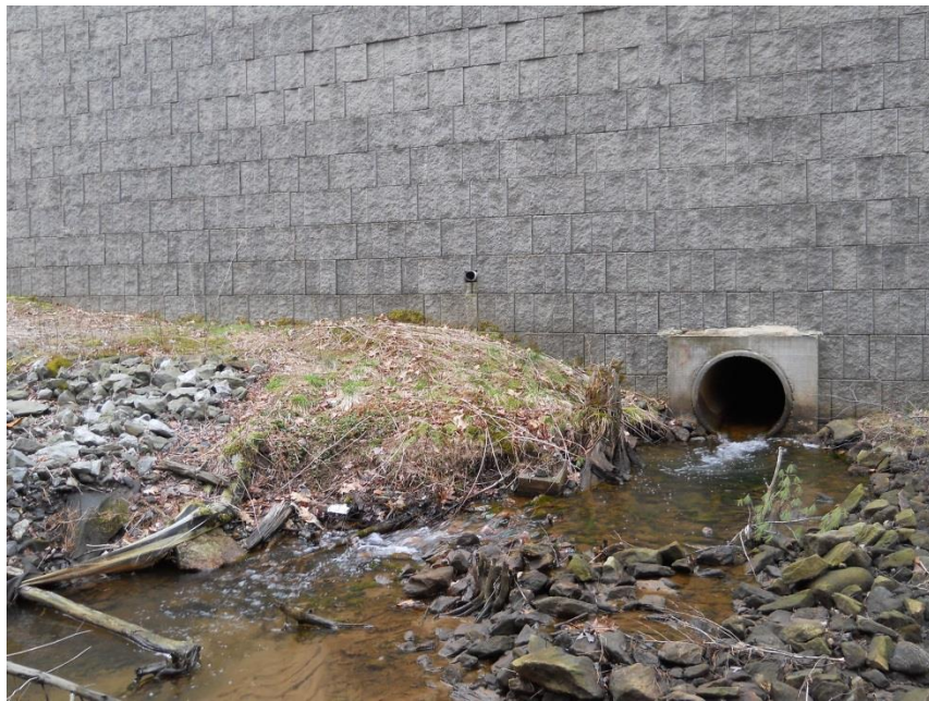
Figure 6: Culvert outlet at opposite end of the crossing seen in Figure 5; note definite channel and rocky substrate.
