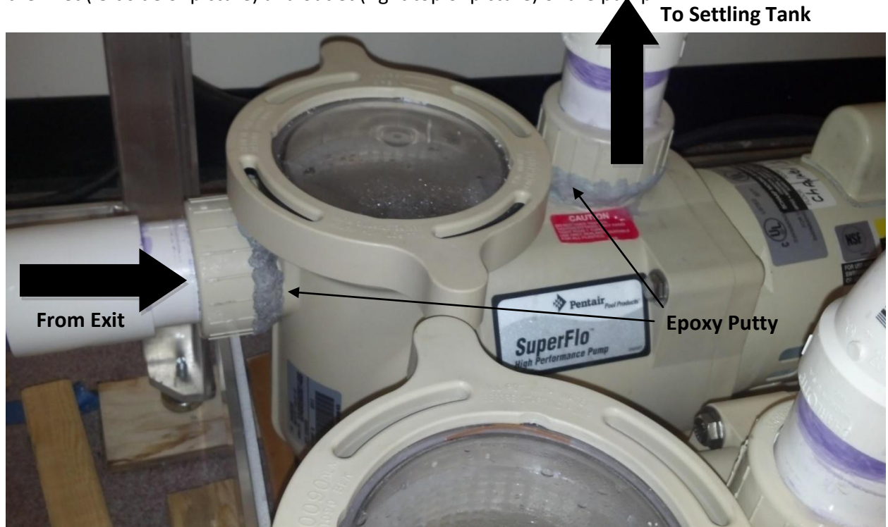
Figure 5. One of the three pumps that push water into the settling chamber of the water channel. Both inlet (left) and outlet (top right) had leaks and were patched using the epoxy putty.
