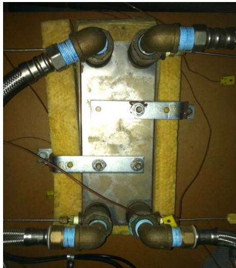
Figure 16: Existing flat plate heat exchanger in the solar thermal system.
