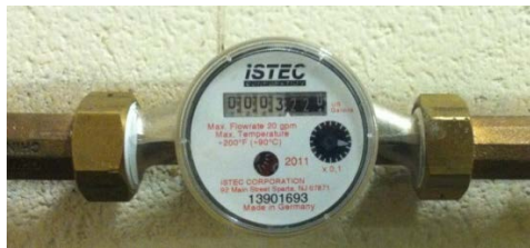
Figure 14: iSTEC 1700 Series Water Meter installed on the boiler water supply.
