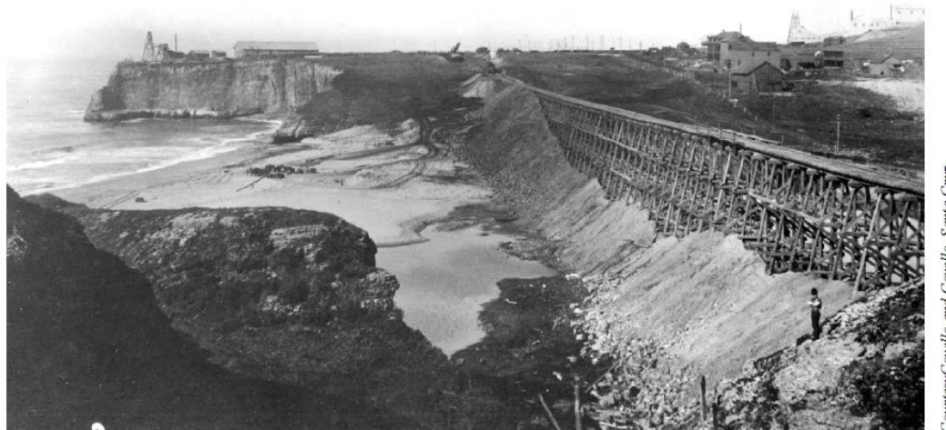
Figure 3.1. Construction of the railroad trestle crossing the mouth of San Vicente Creek at the Davenport beach. (Copied from ESA 2001)
